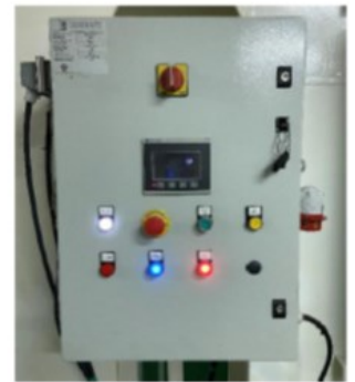
Touch Screen Distribution Panel
