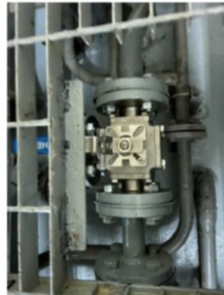
3-way valve from Storage Tank #1
